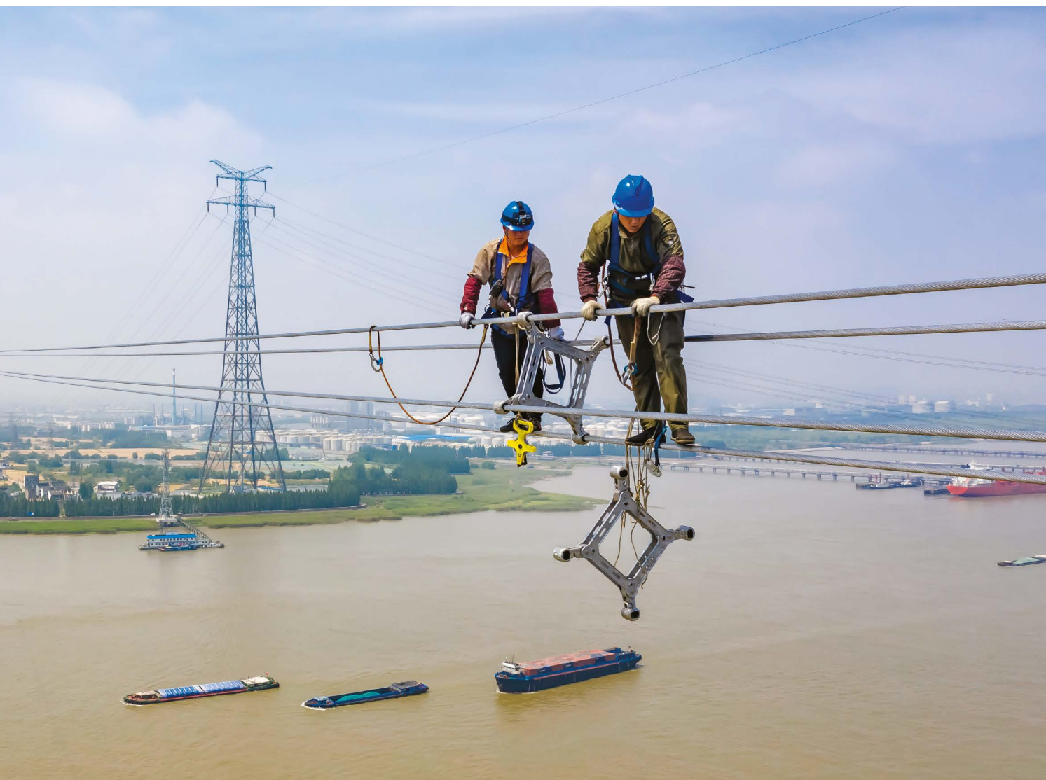
Spanning the Yangtze River with an ultra-high voltage power line exemplifies the scope of China's technological enterprise.
